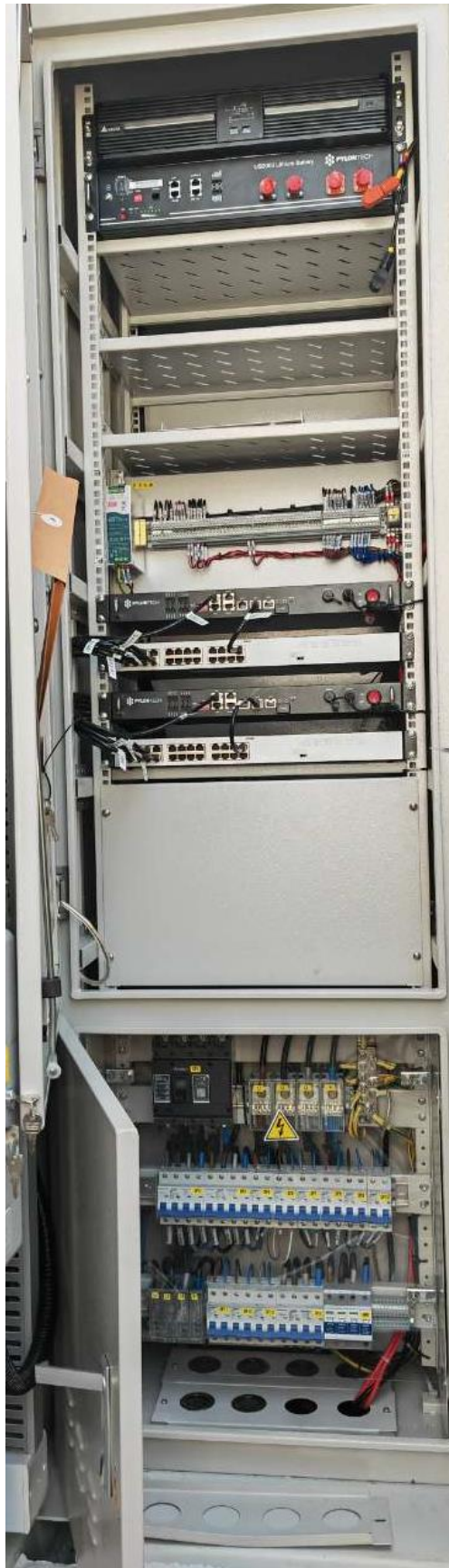
The electrical cabinet contains UPS, MBMS, micro breaks, and secondary electrical schematic diagram is shown in the following figure.
